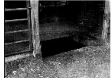
Access point into manure pit where two died after entry, Iowa FACE IA024, 025.
