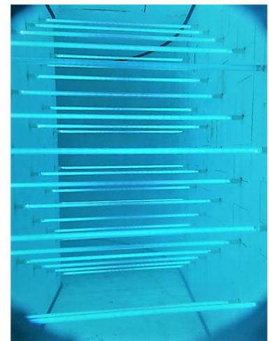
Figure 6. Illustration of the UVC plenum operating in the tRVS, as graphically shown in Figure 5.
